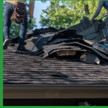
Roofing Contractor Alert
