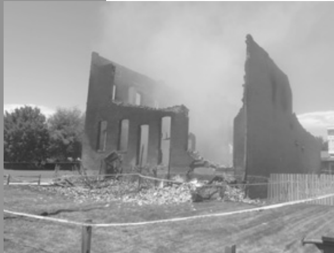
Halls Corner Bar, Genesee, Idaho, taken by Mark Aamodt, Deputy Fire Marshal, Office of the State Fire Marshal
