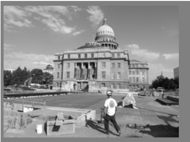
West Wing view of Idaho State Capitol during renovation and addition of underground wings started in 2007. Photos taken by Knute Sandahl, Deputy State Fire Marshal.
