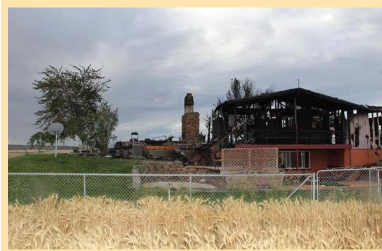
Residential Structure Fire Owyhee County Photo provided by Jeff Sands, Chief Deputy-Investigations
