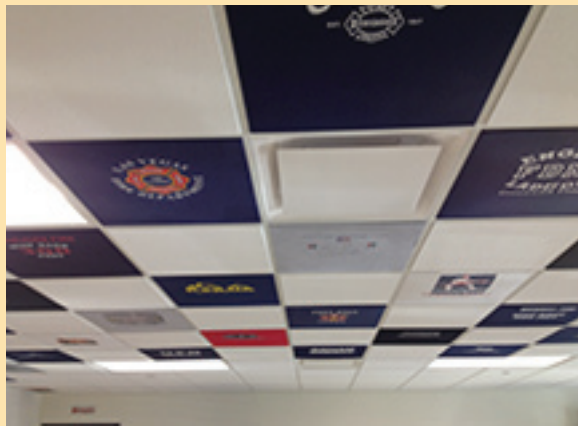
T-shirt Ceiling in Training Room at Rock Creek Rural Fire District Photo provided by Jeff Sands
